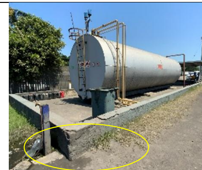
Photo 25 Damaged bund wall
