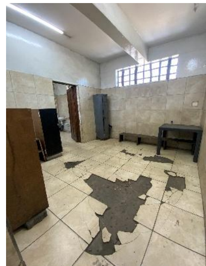
Photo 10 Old Ablution facility not suitable for use. Severely dirty and dilapidated.
